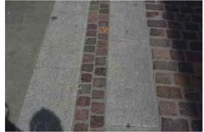
Granite kerb and Porphyry setts, kerbs to be laid flush with paving
