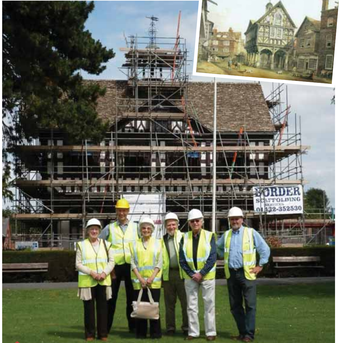
Members of the Friends of Grange Court on a recent visit to see progress on the building including Mayor of Leominster Councillor Eddie Clark. Inset: a copy of a print showing Grange Court when it was in Broad Street, Leominster.
